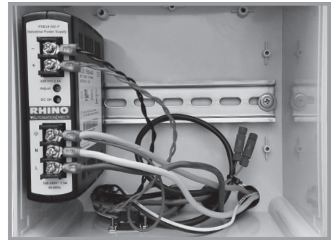
Location of float switch connection leads in controller box.
